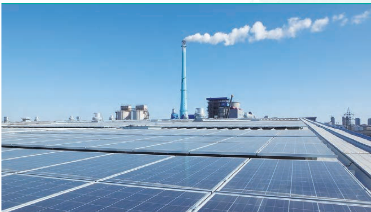
Rongcheng distributed solar power station starts to generate electricity
